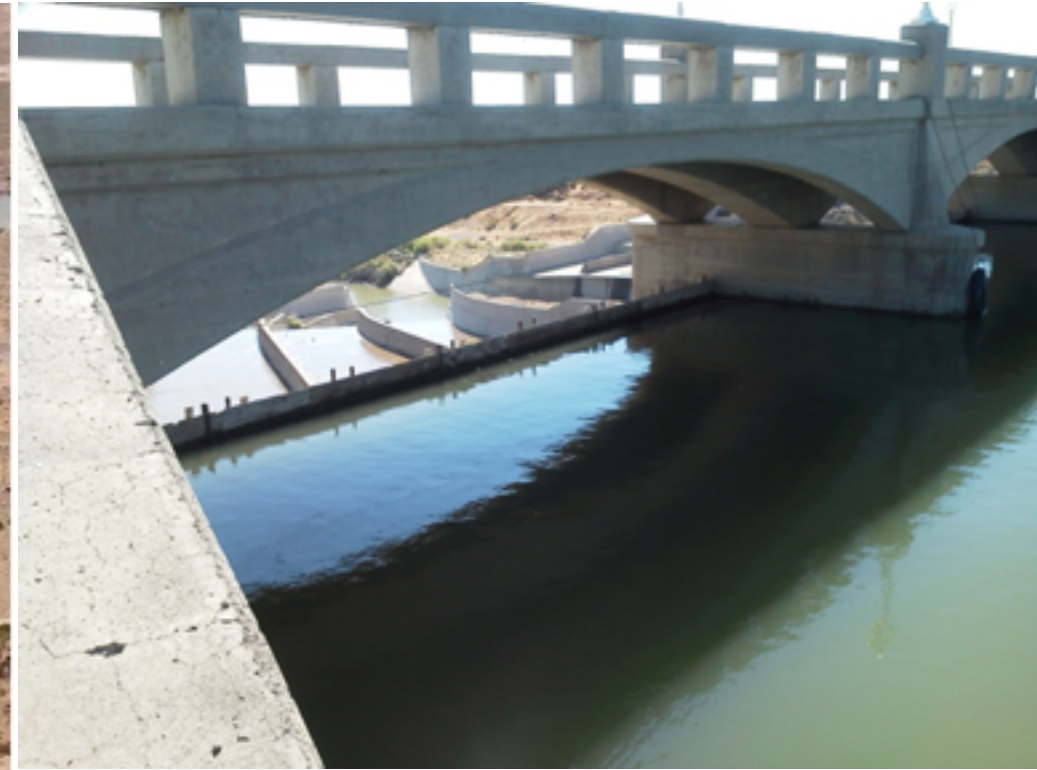
Flashboards installed in 2011
